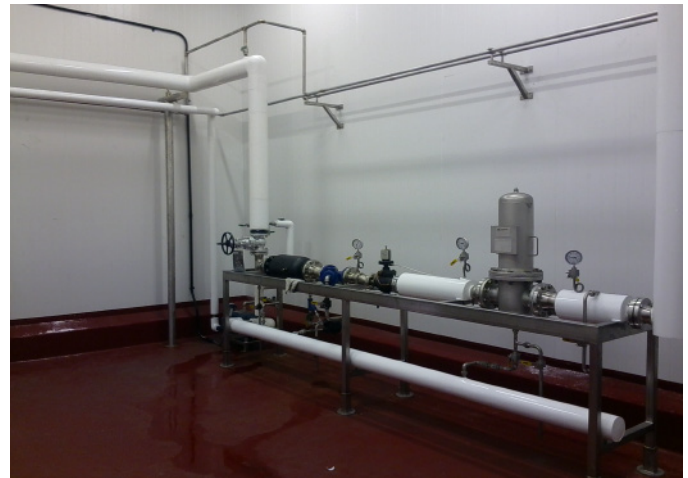
Culinary steam and sterile air systems were provided for this expansion.
