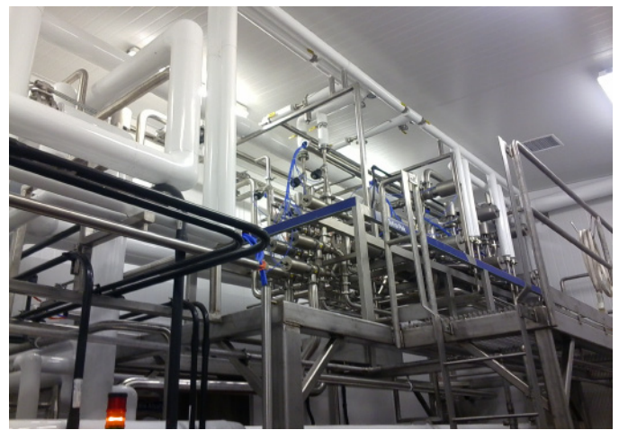
New access platform with end of line valve clusters and steam barrier equipment.
