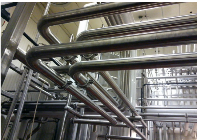
Over 7,000 feet of pipe and tubing were installed much of which was inside existing process areas
