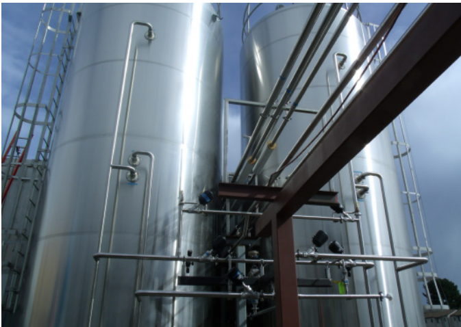
Chilled water piping and product lines installed on the 2 new tanks.
